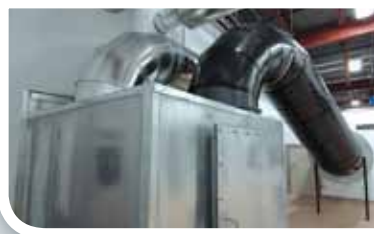
Branch Duct Work
